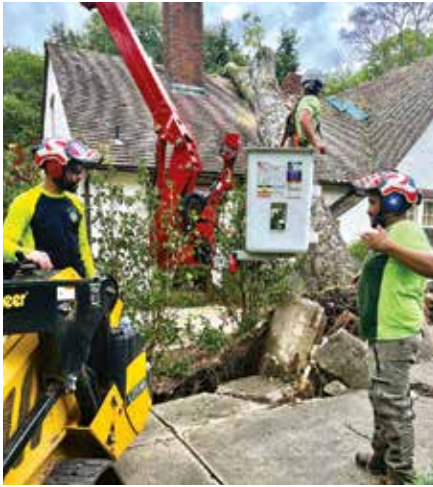
Another uprooted tree finds a resting place on a building, this time a historic home in the Cloverdale area.
